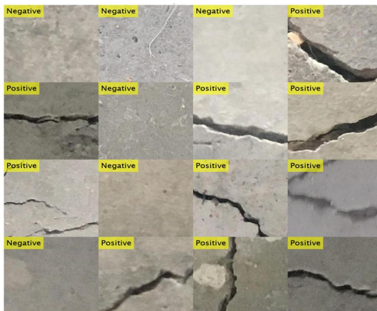
Fig. 3. Classification of concrete crack images
