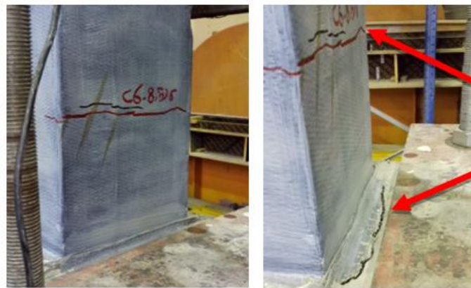
Fig. 13. The cracks of C2C1 column at failure under the lateral load. Separation of the fiber is noticed
