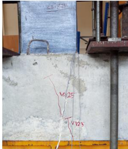
Fig. 12. The cracks of column C2C1 at failure under the ultimate axial load
